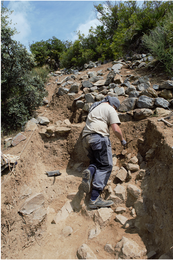
Fig. 32. Detail of the cleaning of the west slope just below the Mesa Redonda summit. Several stones that made part of a wall are spread across it.
