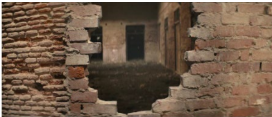
IMG. 90.7, Article 15, Hole in the wall
