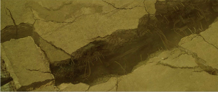
IMG. 31, KPC, Cracks in a bridge
