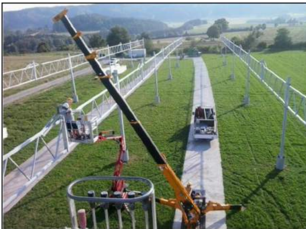
Fig. 4. (Left, source: BayWa r.e.): Installation of APV power plant with mobile soil protection panels in August 2016.
