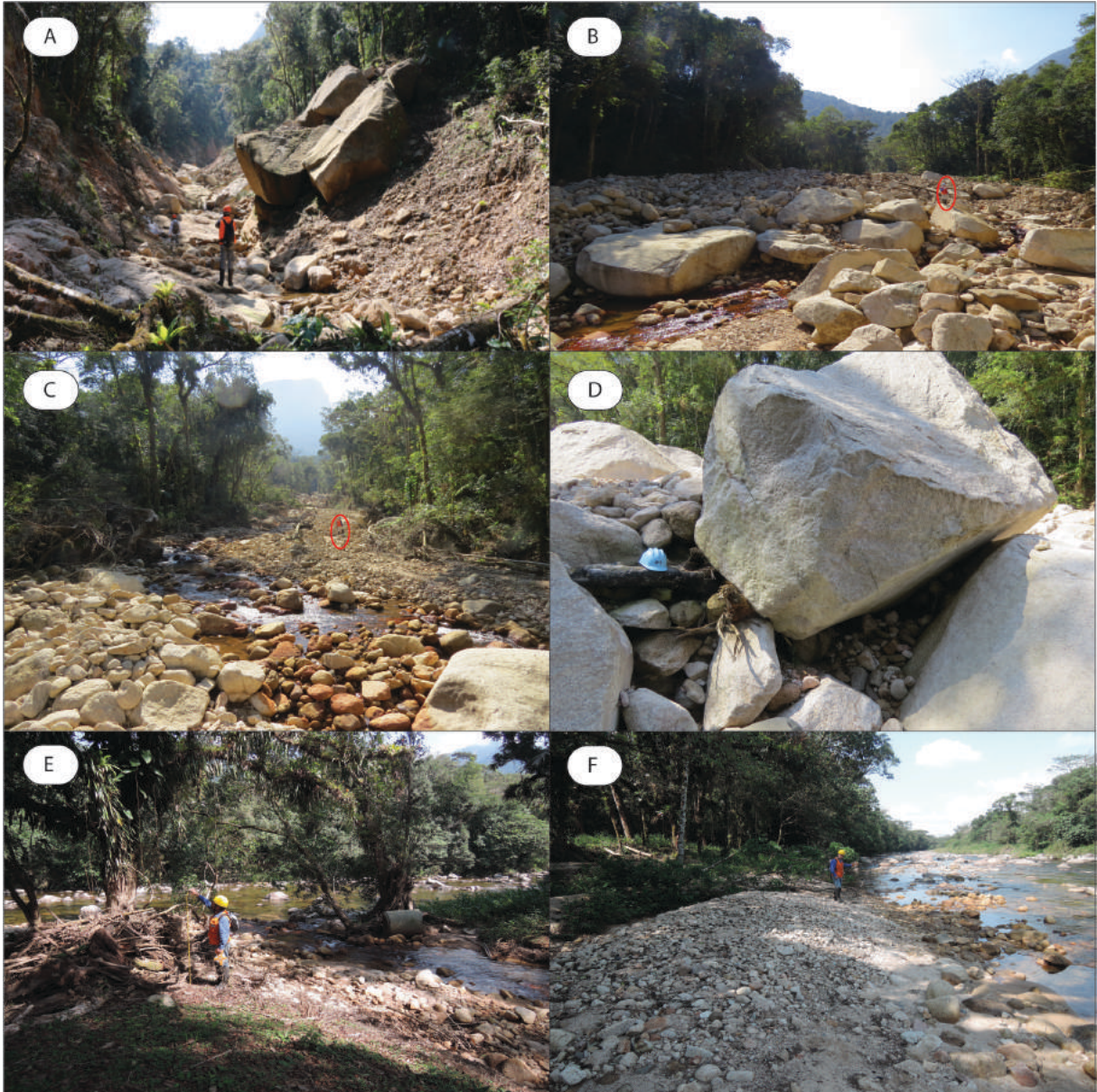
1 2 Figure 6: A) Pronounced erosion and scour of channel bed is observed at the upstream section (SG23) – 1.8 m 3 human profile for scaling. B) Intense accumulation of debris at the middle section (SG13) – in detail, a 1.75 m 4 human profile for scaling. C) Accumulation of debris at the downstream section (SG6), with smaller sized-boulders 5 than in the middle section - 1.75 m human profile for scaling. D) Reversely graded pattern observed in debris dams 6 (SG5). E) Debouchment of the Pedra Branca river into the São João River, where flow height reached up to 2 m. 7 F) São João river, which received sediments from the Pedra Branca debris flow (photo from August 2017).
